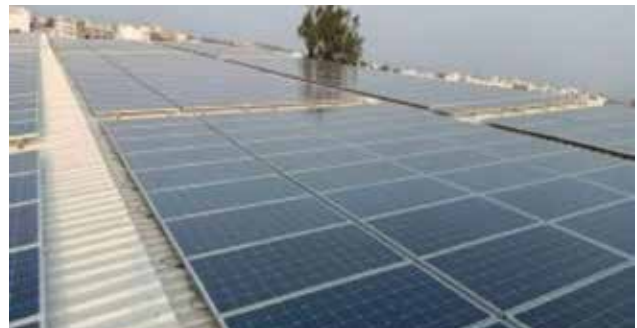
Initiative to use renewable energy in factory premises
